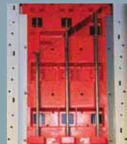
Isolated/insulated vertical bus assembly
